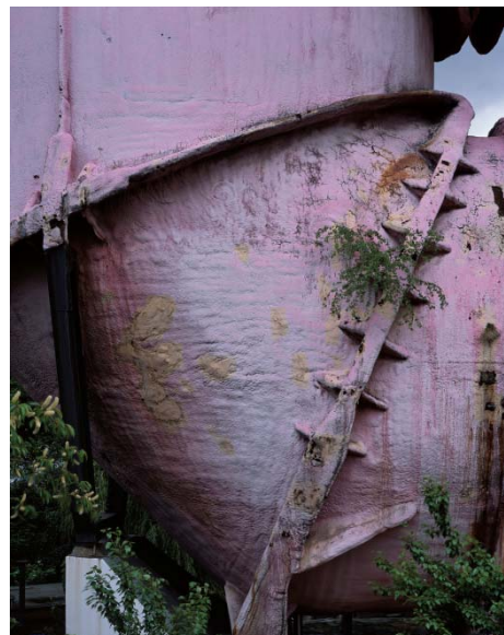
H el ene Binet: Ludwig Leo, Circulation Tank of the Hydraulics Laboratory, Berlin (Germany), 2014   H el ene Binet
